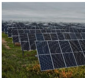
Ground-mounted solar plants
